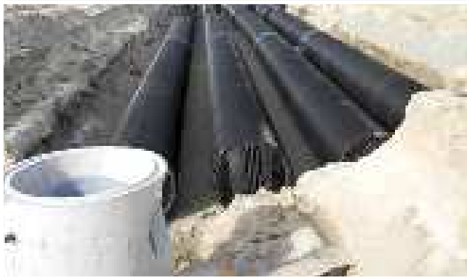
CDS pretreats a rainwater harvesting cistern.
